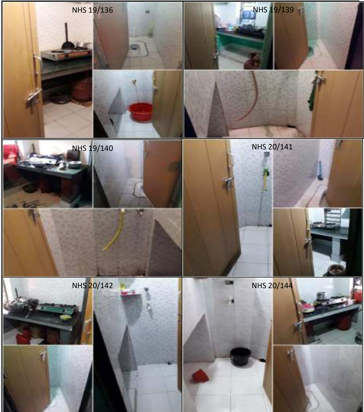
INSIDE BLOCK REPAIRING WORK OF NHS QUARTERS AT R N COLONY OF SONEPUR BAZARI AREA
