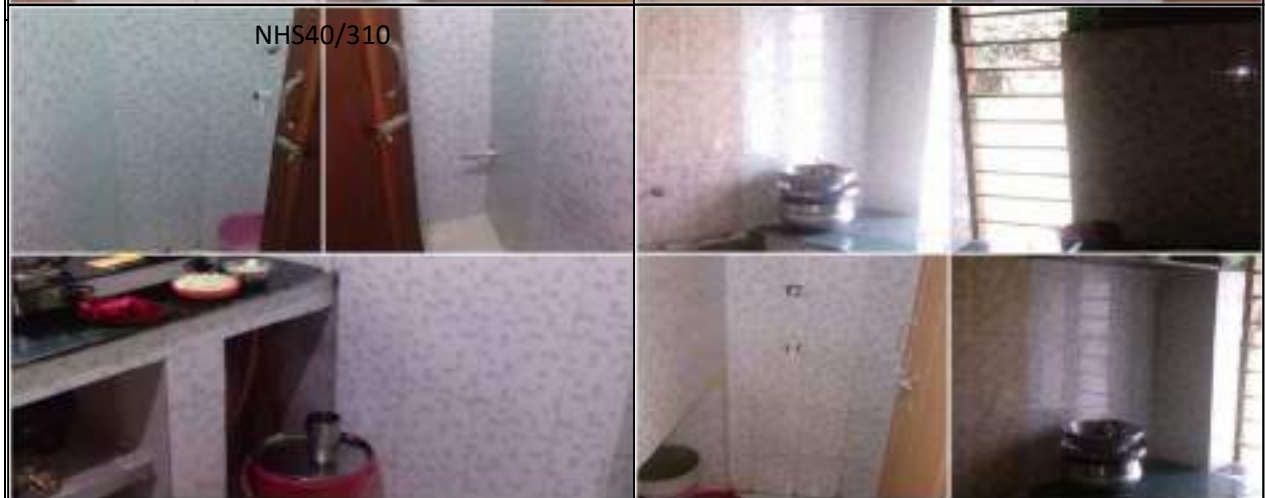
INSIDE BLOCK REPAIRING WORK OF NHS QUARTERS AT R N COLONY OF SONEPUR BAZARI AREA
