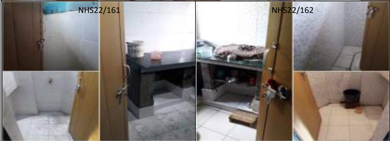
INSIDE BLOCK REPAIRING WORK OF NHS QUARTERS AT R N COLONY OF SONEPUR BAZARI AREA
