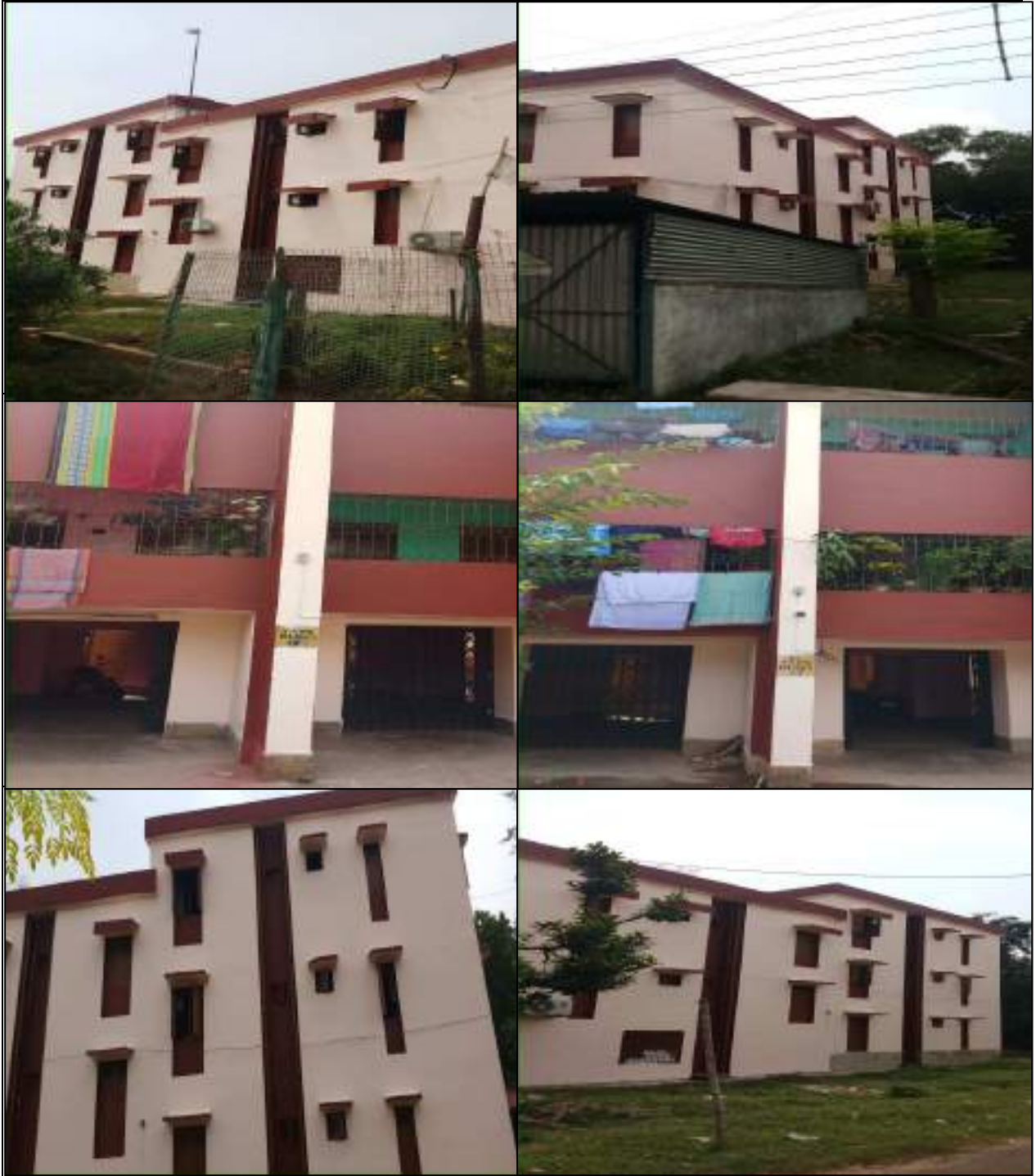
BLOCK REPAIRING WORKS OF B TYPE QUARTERS AT R N COLONY OF SONEPUR BAZARI AREA
